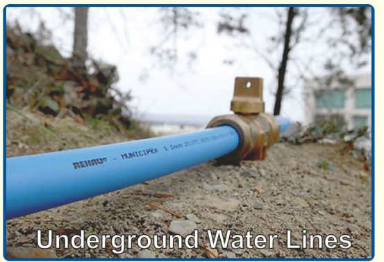
Underground Water Lines
