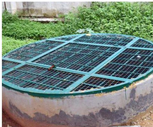
Rain water harvesting pits in common areas
